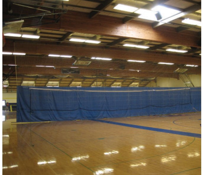
Newberg High School: Limited ceiling height in gymnasium
